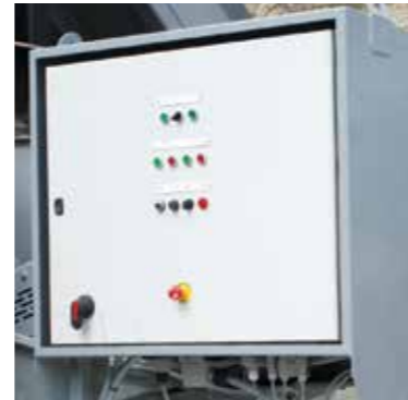
H12 Feeder Control Panel
